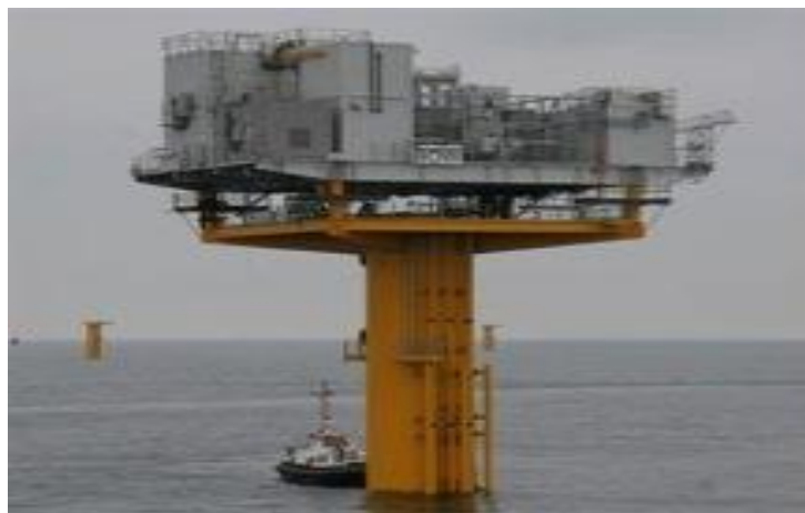
Figure 18. An Electric Service Platform (ESP) for an offshore wind facility [29]
